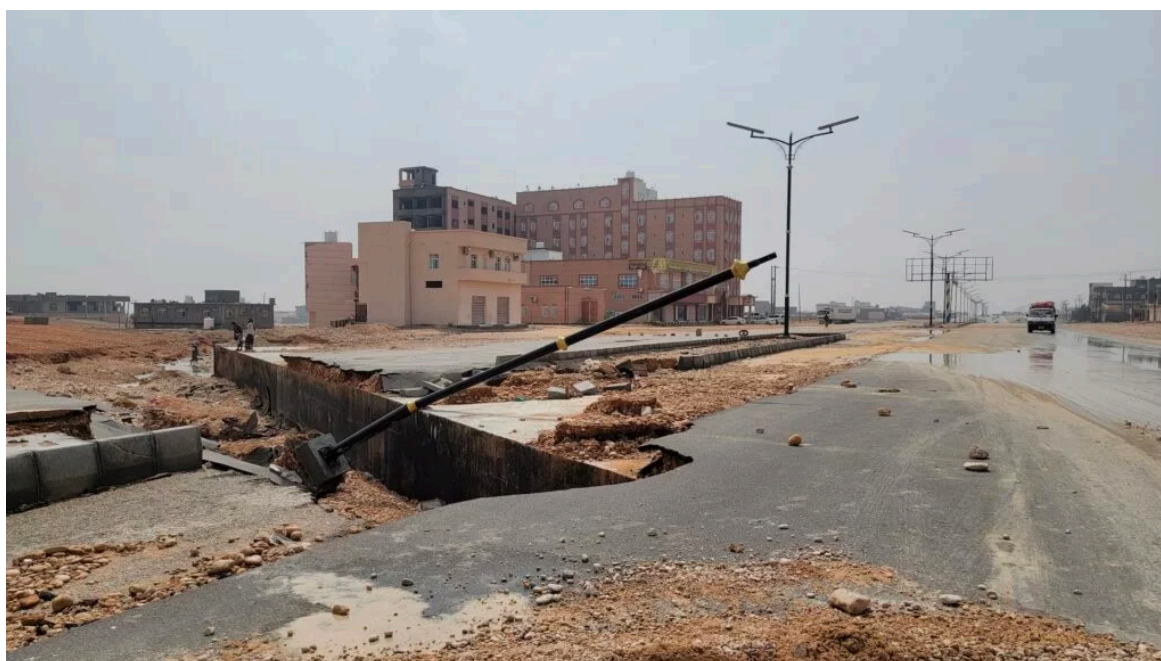
Destruction on a street in Al-Ghaydah city on October 25, 2023, as a result of Cyclone Tej // Sana'a Center photo by Moaz Nasser
